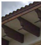
9 WOOD OUTRIGGERS BROWN TEAK WOOD REF. MATCH EXISTING SHIPPING CENTER REF. COLOR CUSTOM BROWN SEE 3/A-400
